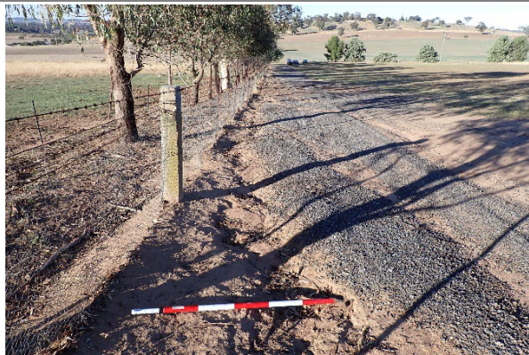
Plate 8-2 View to the south in the southern portion of the Project Area showing evidence of slope wash erosion along the proposed access track for the BESS site.
