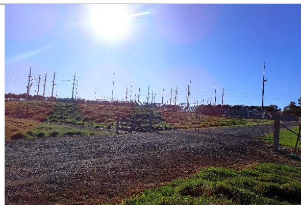
Plate 8-6 View to the north east in the northern portion of the Project Area showing the existing substation.
