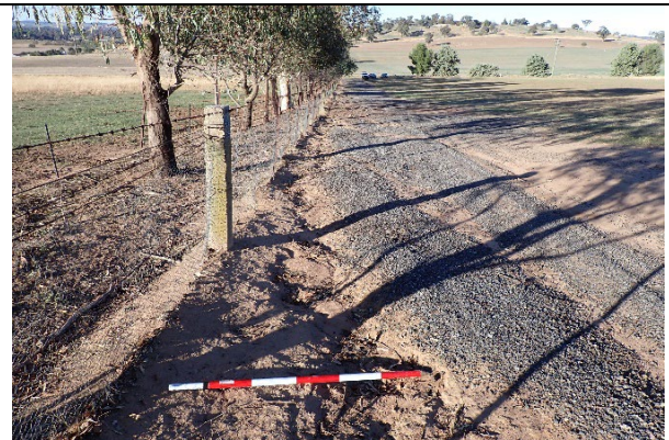
Plate 4-2 View to the south in the southern portion of the Project Area showing evidence of slope wash erosion along the proposed access track for the BESS site.
